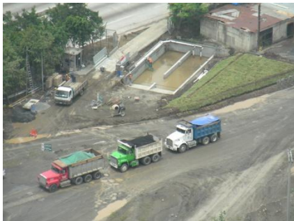
Over view Model 400 Quick with 30,000 Gallon Solid Separation and Water Recycling System
