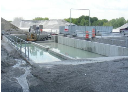
Dual Drive Down Solids Settlement and Water Recycling Area for 2 MobyDick Wheel Washing Units
