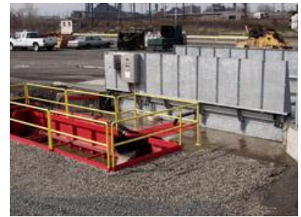
Moby Dick Unit is installed with a Frutiger Recycling Tank
