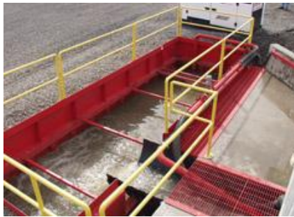
Wash-water return from the wheel washing unit into the 5000 Gallon Recycling Tank.
