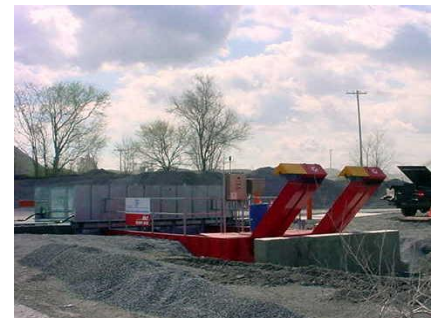
Dual scraper conveyor automatically dewateres and removes solids.
