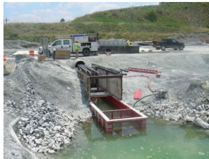
Common drive down solids separation and water recycling area with control panels & flocculent system.
