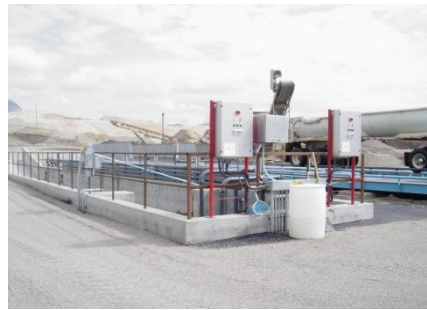
Common Drive Down Solids Separation and Water Recycling Area with Control Panels & Flocculent System.
